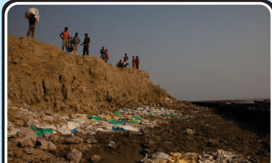
Futile effort to repair embankment, Sagar island
