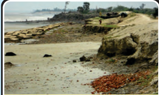
Erosion of embankment at Mousuni island, Namkhana block, Sundarban
