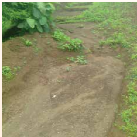
Trench filled with eroded top soil
