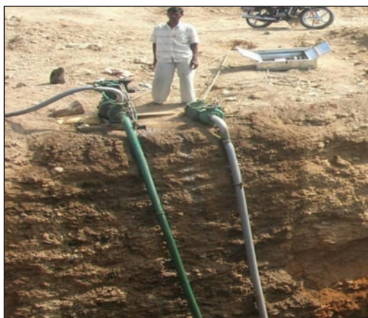
Diesel pump set
