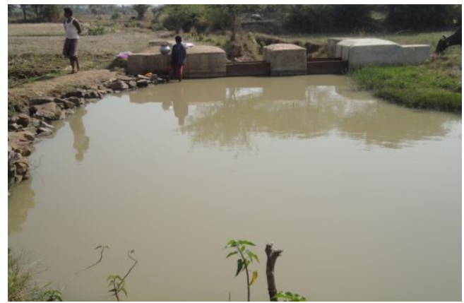
Check dam - Tahkapal, Bastar district, Chattisgarh
