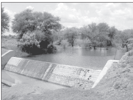
Fig. 15 : A masonry check dam at Kothapally watershed, Ranga Reddy, Andhra Pradesh, India.
