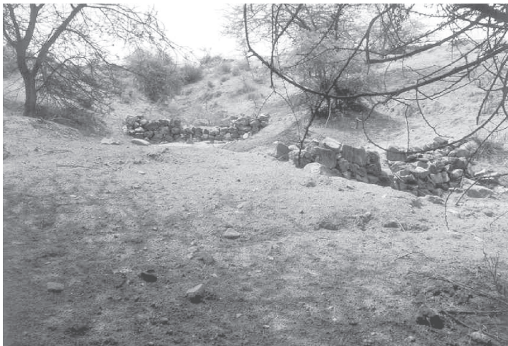
Fig - 7. A series of loose stone check-dams (LSCD) at gully in Jhanwar Watershed (Jodhpur)
