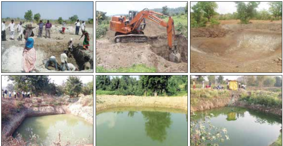
Fig 7. The work undertaken for construction ponds and water stored in ponds at various places in cluster
