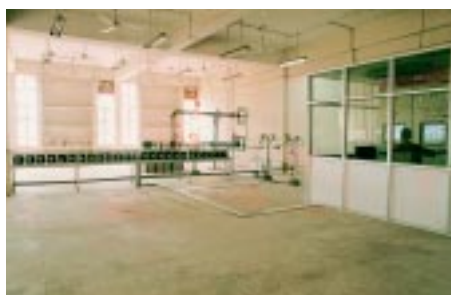
Automatic pump and dripper testing facility are operated by the SCADA
