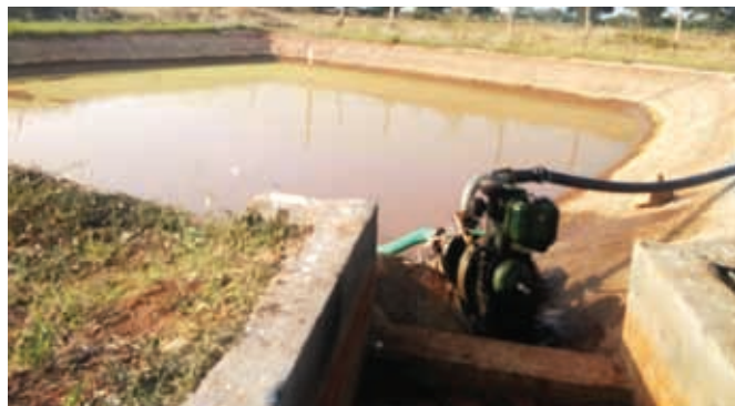
Harvested rainwater in farm pond with lifting pump
