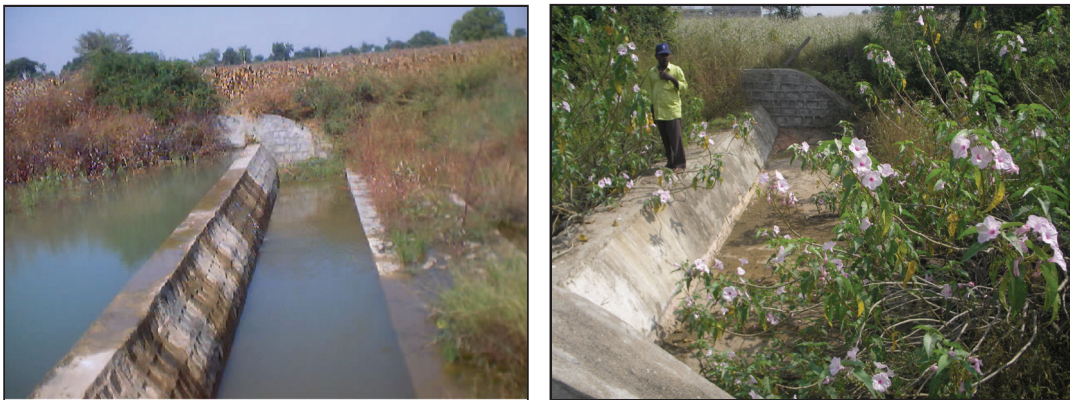
Photo 1: Effectiveness of check-dam in 2006 in Pamana village, Chevella mandal, Rangareddy district and impact of drought in 2009
