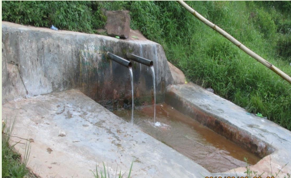
Community Spring Tapped Chamber for Drinking Water at Lumsophoh under Umsarang IWMP-I GPS Reading: N-25°40'02.1"::: E- 92°59'19.4"
