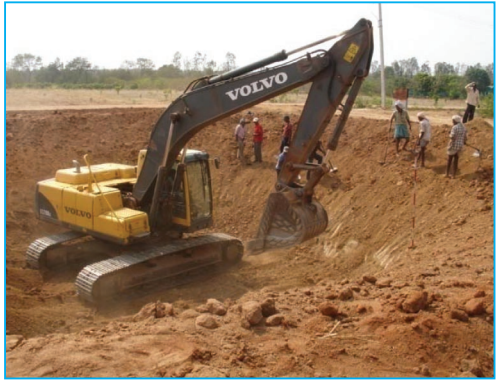
Fig18. A view of earth excavation with V 200 model in dugout farm pond
