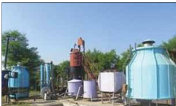
100 -kW biomass-based power plant
