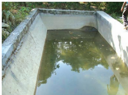
Fisheris started in the Pucca structure (water storage tank for supplemental irrigation)
