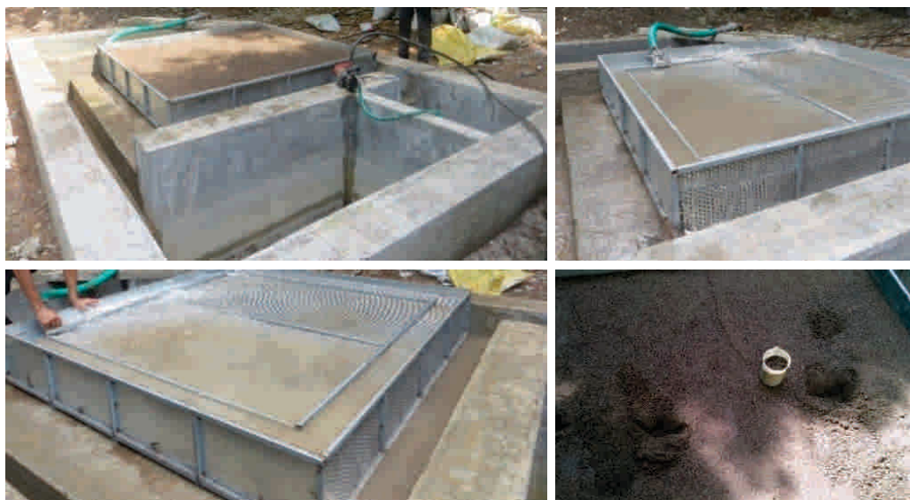
Plate 3.1.4. View of the online screen-gravel filter
