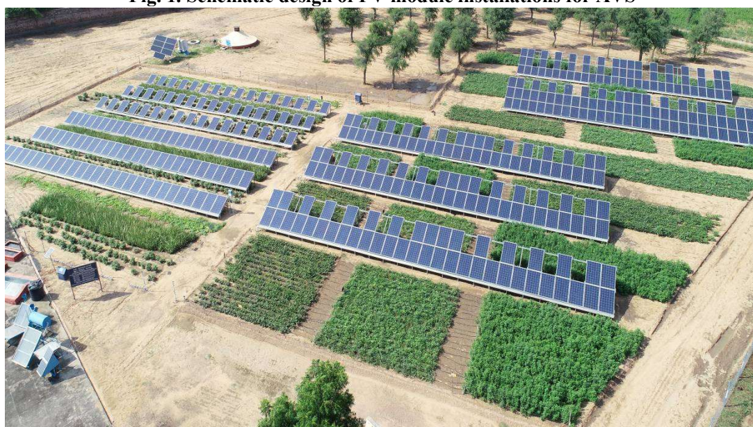
Fig. 2. Installed agri-voltaic system at ICAR-CAZRI, Jodhpur, India
