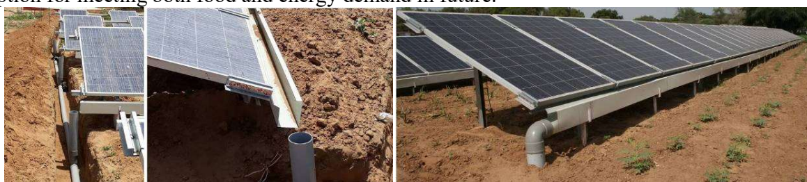
Fig. 6. Rain water harvesting system from top surface of PV module
