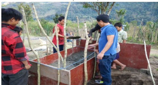
Fig 8 Transfer the mixture into the same wooden box to make it 0.4 ft thickness above the base of supporting structure
