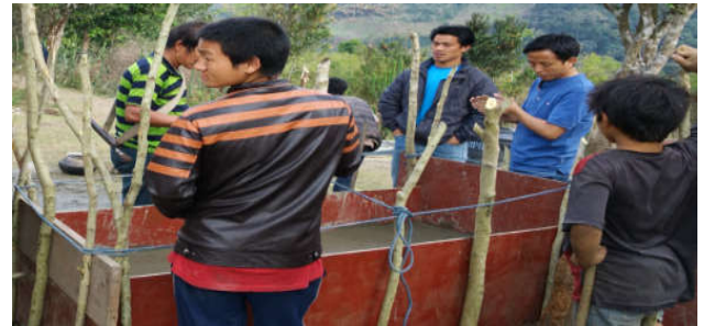
Fig 10 Keep it without disturbing for 7 days for proper setting of cements and other ingredients
