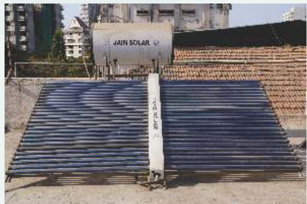
Fig. 15.6 Rooftop Solar water heater
