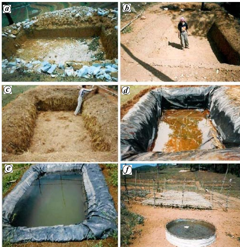
Figure 2. Different stages of Jalkund preparation. a , Excavation of Jalkund . b , Plastering with clay. c , Cushioning with pine leaf. d , Lining with LDPE black agri-film. e , Rainwater collected in Jalkund . f , Thatch cover to prevent evaporation.
