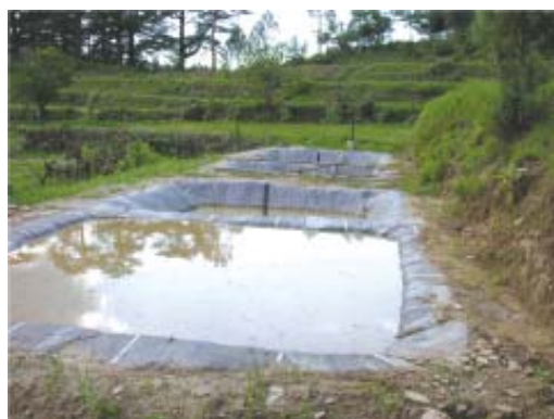
LDPE lined tank for Runoff harvesting
