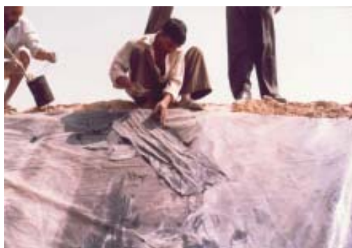
Fig 5b: Repairing of the puncture film by pasting small piece of film with the help of butamin.
