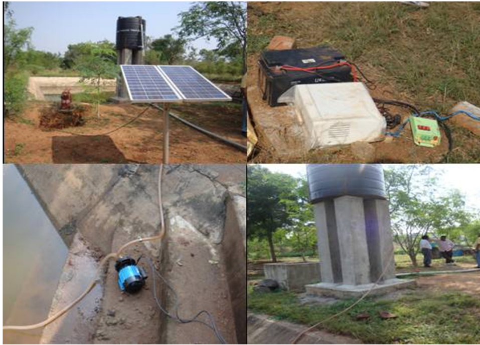
Fig. 2. Pictorial view of different components of developed irrigation system.
