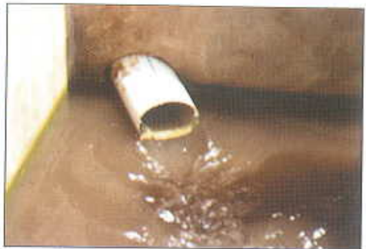
Photo-14 : Collection of spring water in to a cement tank from ridge line of watershed
