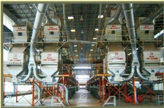
Intermittent four point Lint cleaner trash waste collection system
