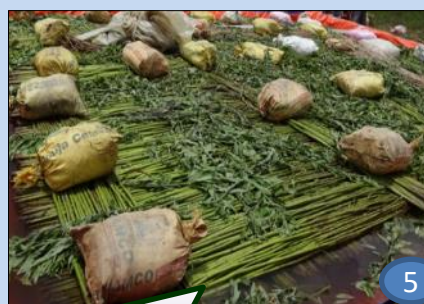
5. Application of load (sand/stone/soil etc.) in cement bag over the jak to submerge the jak
