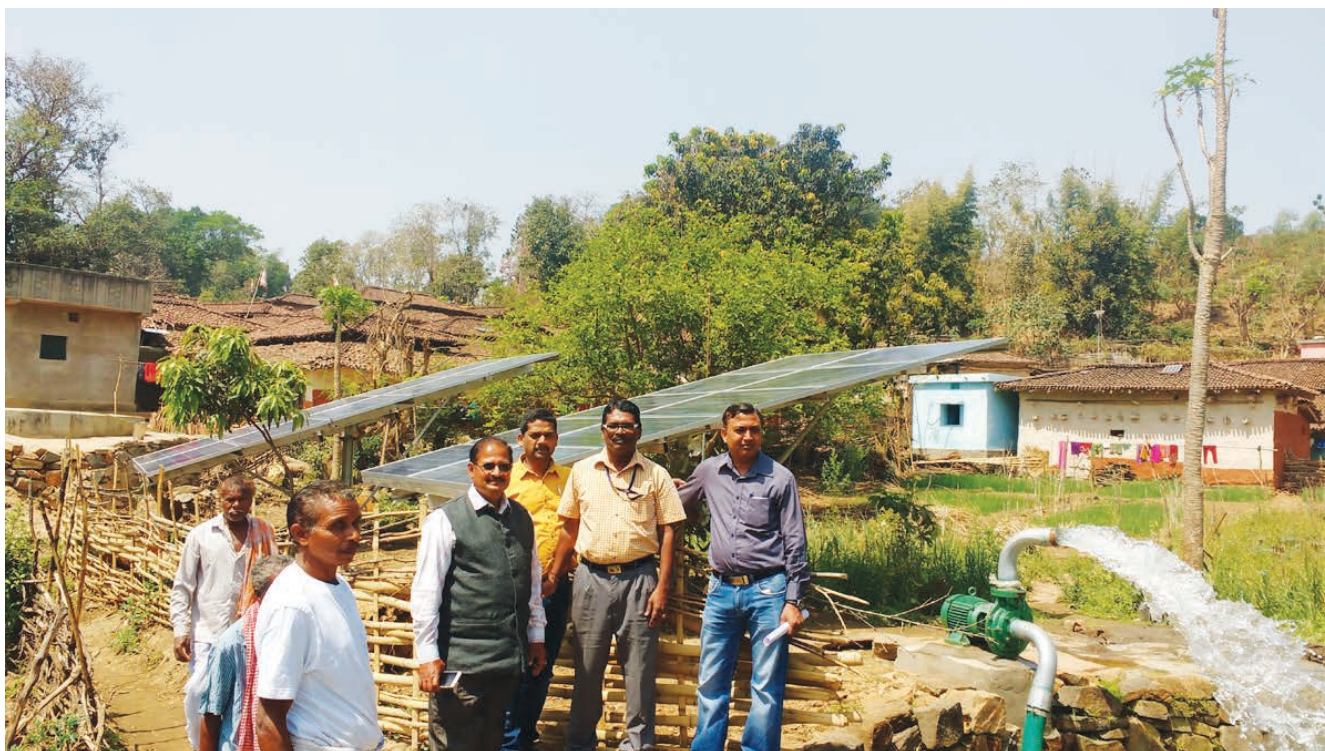
Photo 93. Solar pumpset at Burahkocha village, Ranchi district of Jharkhand
