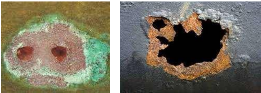
Pitts formed as a result of corrosion
