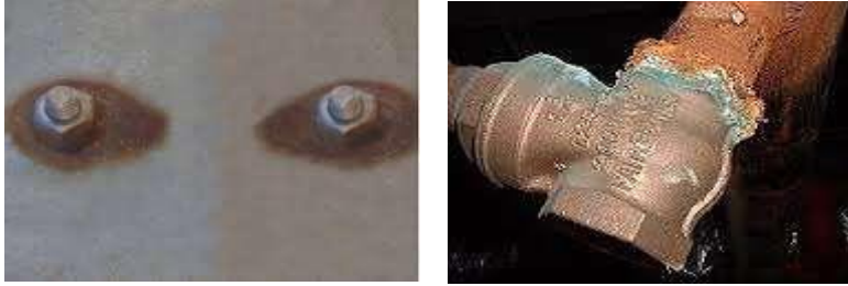
Examples of galvanic corrosion.
