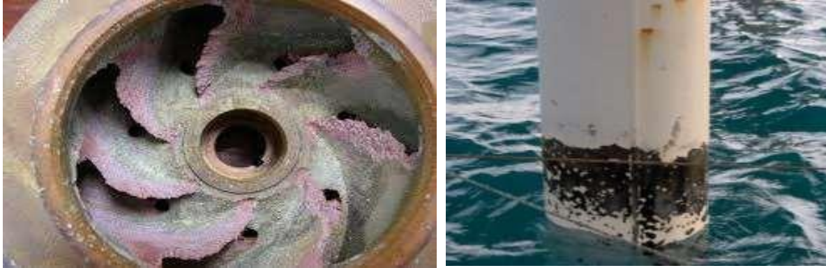
Corrosion of structures in contact with fluid
