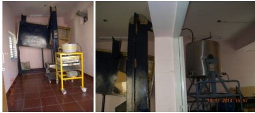
Conveyor system for grain storage and grain boiler
