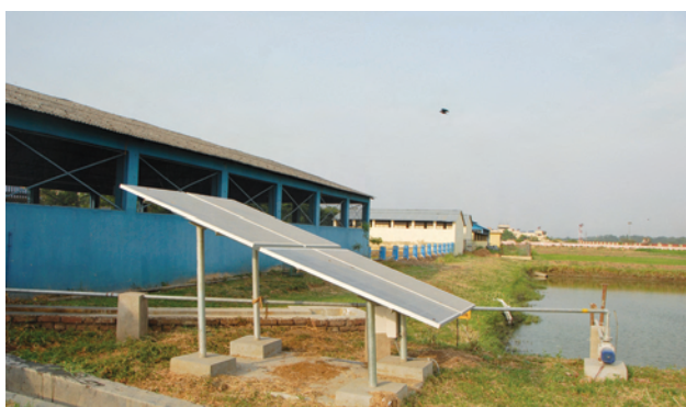
Fig. 113. Solar photovoltaic system for animal shed
